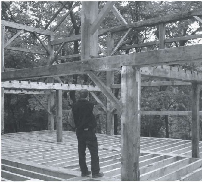
Fig. 6. Knee braces can effectively widen a support and stiffen beams, helping to transfer loads to posts.
