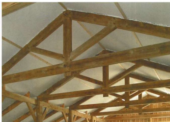
Fig. 17. Typical modern kingpost truss with diagonal web members to support rafters. White oak 6x12 rafters and tie beams span 30 ft.
