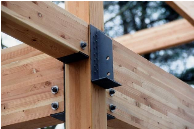
Figure 3 Connection hardware is shop fastened with timber rivets and field bolted. The beam reaction is resisted in bearing on the seat and the bolts are not taking load.
