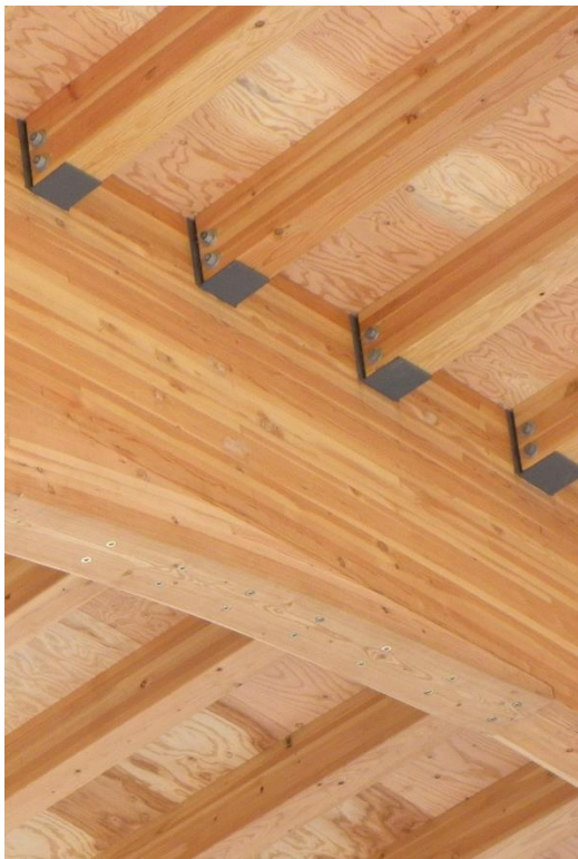
Figure 13 Stiffened seat connections with the bottom of the seat plate exposed
