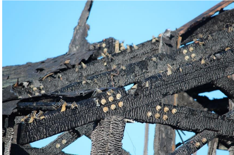
Figure 12 Fire damaged timber structure
