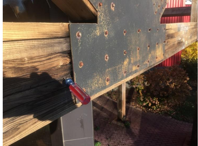
Figure 9 Timber in contact with exposed gusset plate is prone to decay
