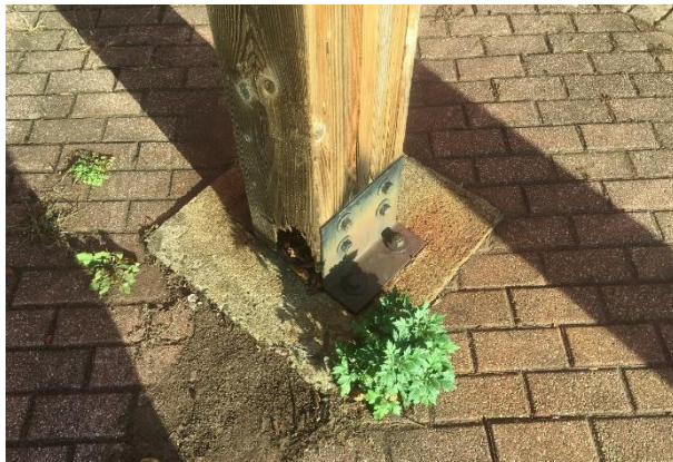
Figure 10 Rotted post base
