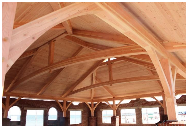
Figure 1 A glulam timber structure with traditional joinery and a CLT roof deck
