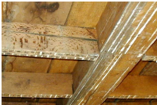
Figure 2 - Failed Butt-Cog Joint
